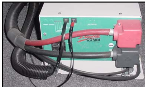
Figure 7-16. Automatic Transfer Switch
