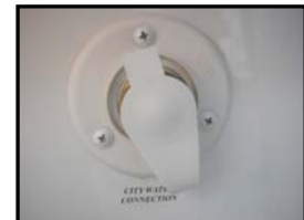
Figure 11-6. City Water Inlet
