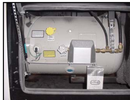
Figure 2-4. Liquid Propane Tank
