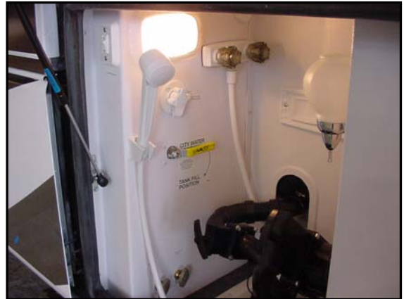
Figure 11-12. Exterior Shower and Exterior Light
