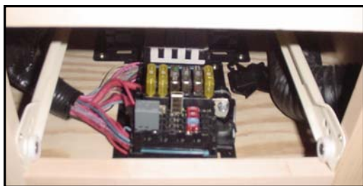
Figure 7-21. Fuse Blocks within Center Console
