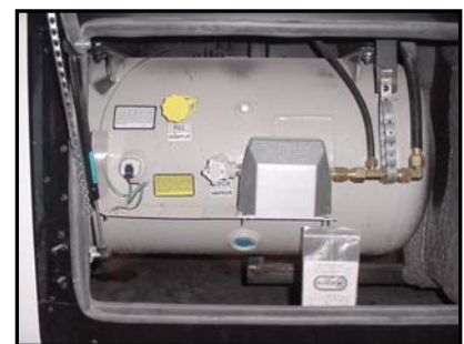
Figure 3-4. Liquid Propane Tank
