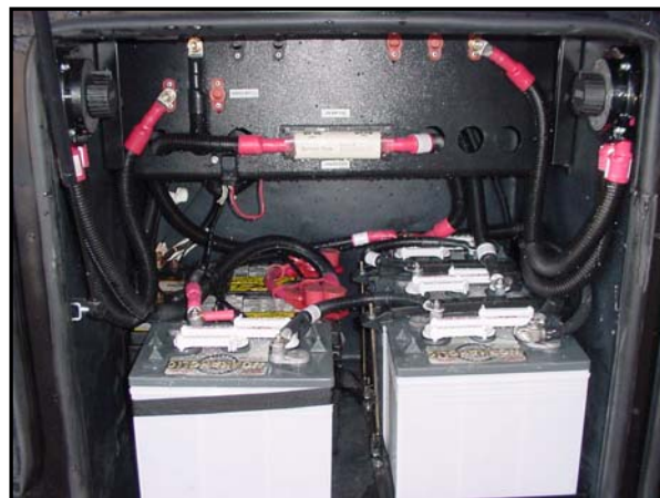
Figure 7-5. 12 VDC Battery System
