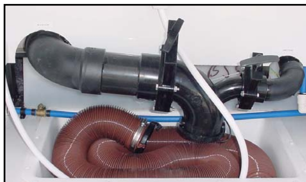
Figure 11-11. Sanitation Coupling, Valve, and Hose
