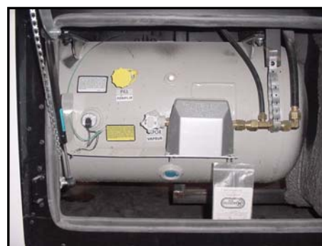
Figure 2-2. Liquid Propane Tank
