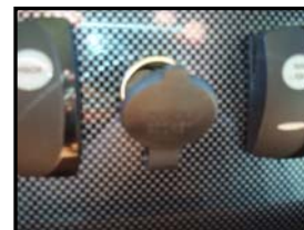
Figure 7-6. Typical 12VDC Receptacle (Bottom)
