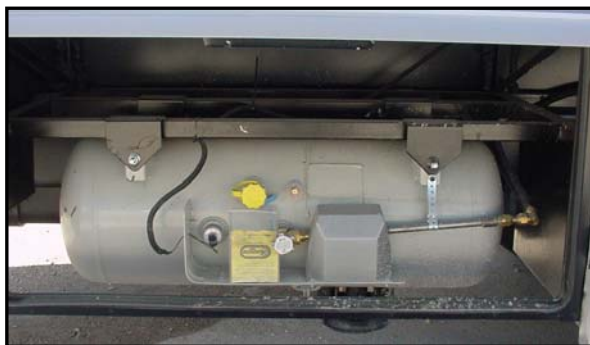
Figure 2-4. Liquid Propane Tank
