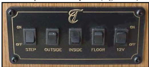
Figure 7-4. Battery Disconnect Panel
