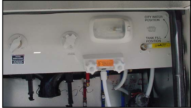
Figure 11-6. City Water Connection
