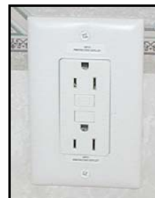
Figure 7-5. Typical AC Receptacle
